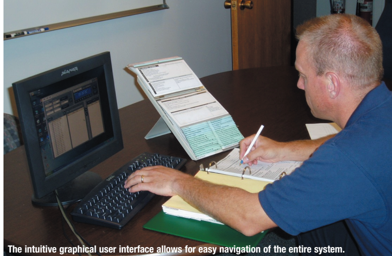
The Eventide installation at CenCom.
