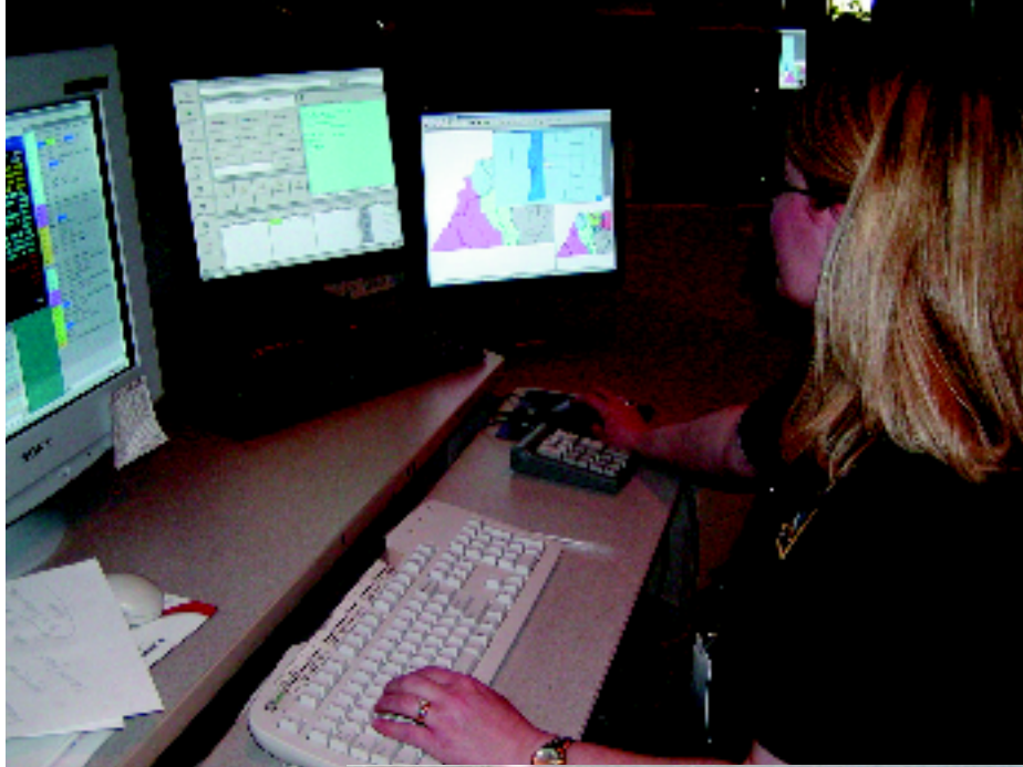
On the Call Dispatcher Cari Parkinson relied on her VESTA 9-1-1 system's programmed auto dial to transfer calls to specific groups for dispatch and information processing. Transferring lesser-emergency calls and calls for information to designated groups helped reduce ring and hold times for emergency calls.
